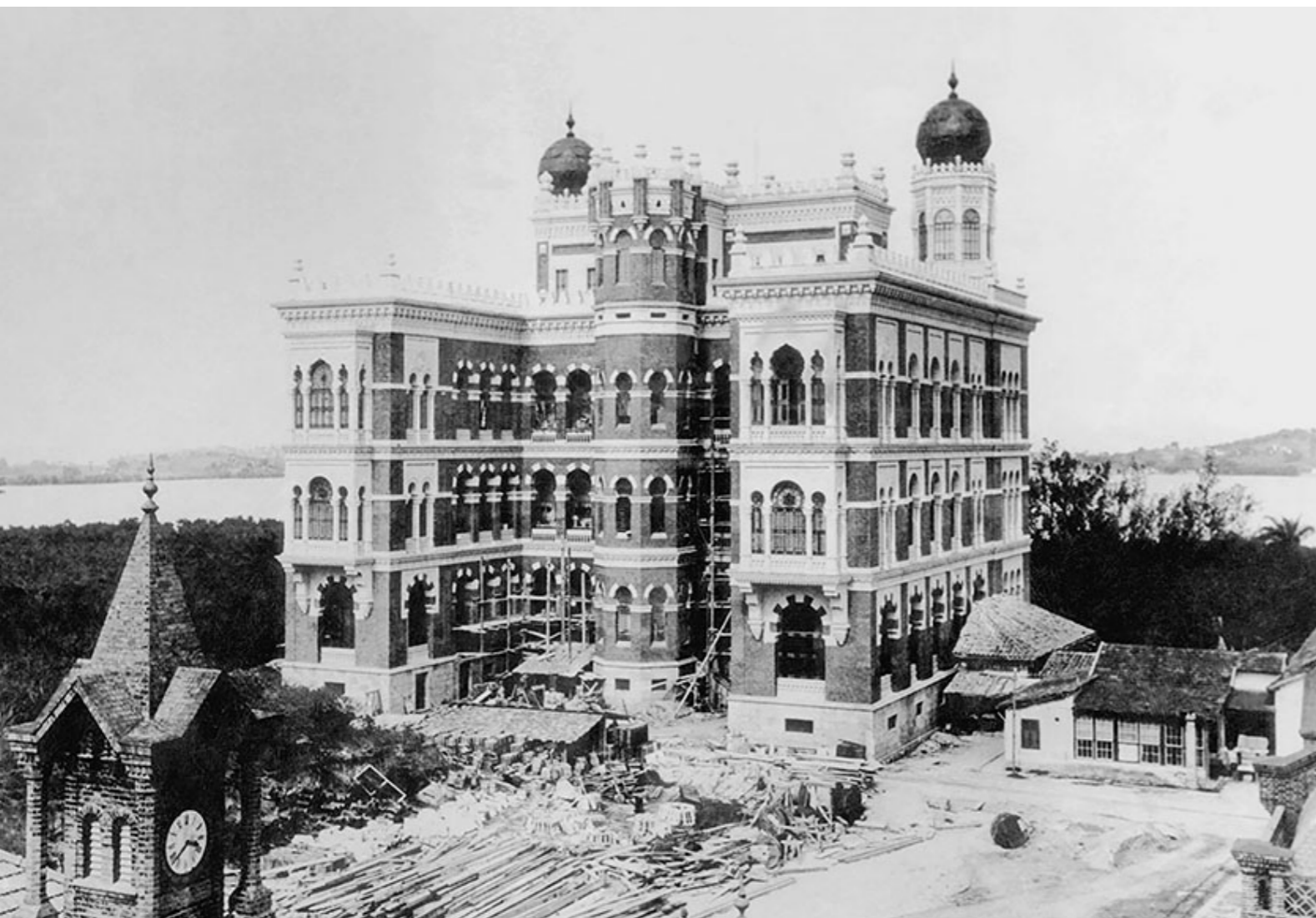
Moorish Pavilion under construction and, on the left, a detail of the tower of the Plague Pavilion 1907
