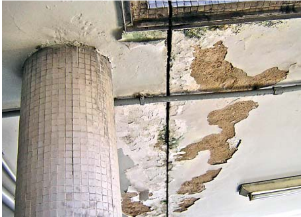
27 – Infiltração das lajes – Leaking roof
