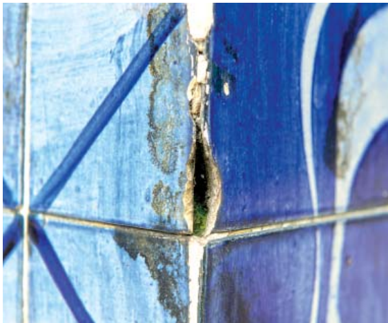
39 – Fissura na parte central do painel – Crack in the central part of the mural
