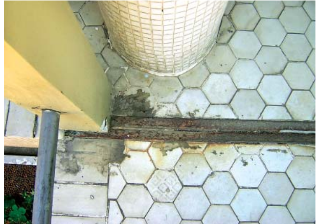
28 – Junta de união entre os blocos – Joining section between the two blocks
