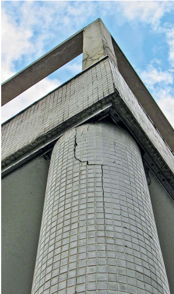
29 – Exemplo de fissura na coluna – An example of a crack in the pillar
