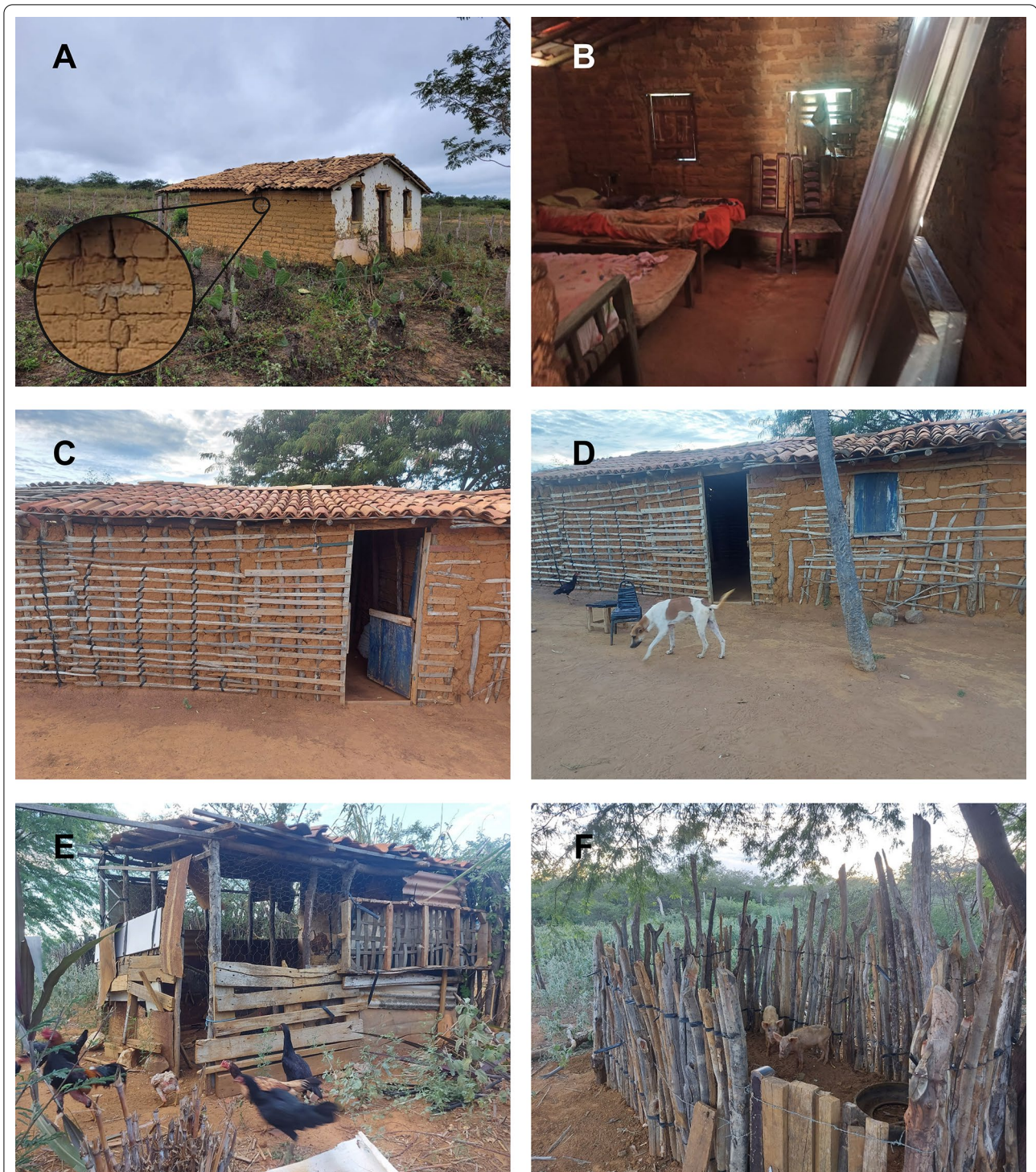
Fig. 2 The epidemiologic scenario of poor rural communities in many Latin American countries. Mud house with cracks where triatomines can hide (A–C), with detail of a crack in a rural adobe/brick house (A). B Inside of the house illustrated in (A). Mud house with cracks (C) with presence of domestic animals in the environment: dog (D), chickens (E) and pigs (F). These animals can attract triatomines for a blood meal, thus helping maintain the peridomestic cycle of T. cruzi . Photographs were taken in rural areas of the municipalities of Tremedal (A and B) and Irecê, Bahia, Brazil (E–F)
