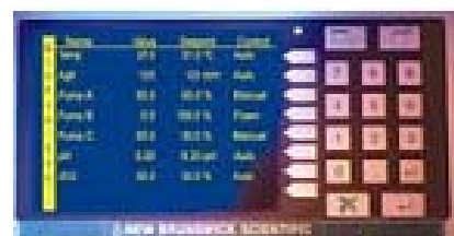
Painel de Controle
